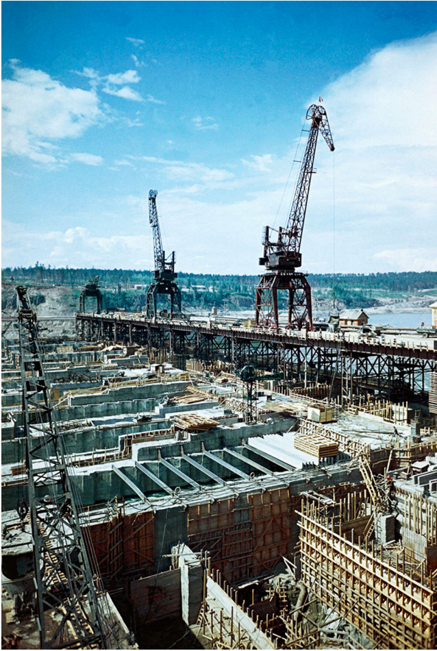
Fig. 28. Building the Bratsk Hydropower Plant, 29 September 1959. © RIA Novosti archive, image #315182/Michael Trahman/CC-BY-SA 3.0.
